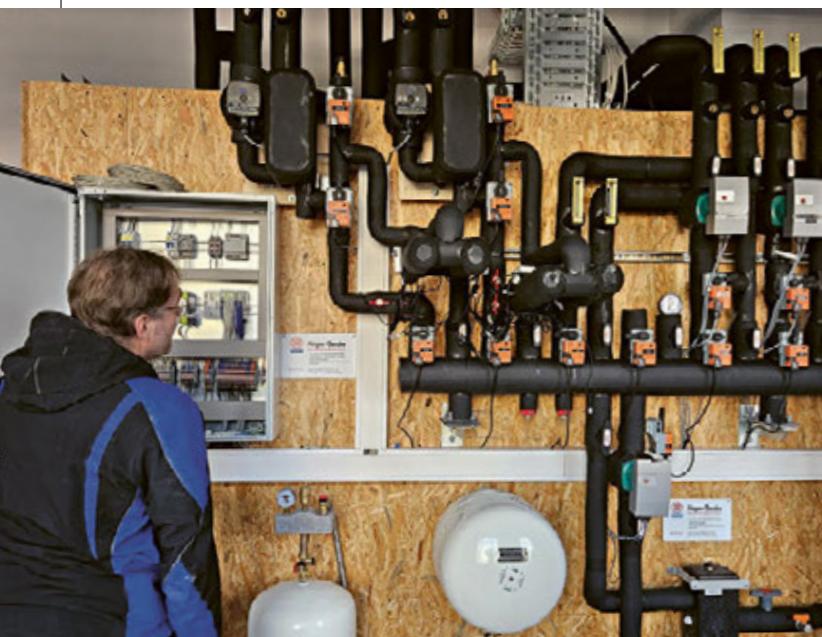
THE DISTRIBUTION POINT ensures the optimum mix of heat media in the energy system as a whole.
