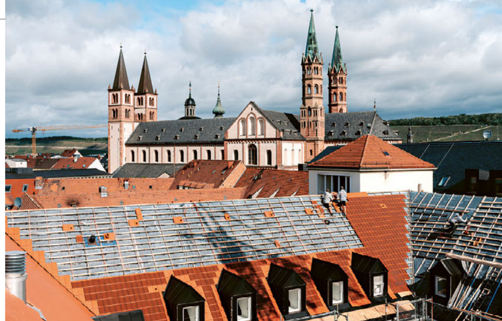
A SIMILAR APPROACH: Photovoltaic system in keeping with landmarked building standards on the roof of the convent of the Congregation of the Sisters of the Redeemer in Würzburg. With the help of specialists for energy-conscious construction from the Bavarian State Office for Monument Protection (BLfD), the entire convent site is being refurbished.
